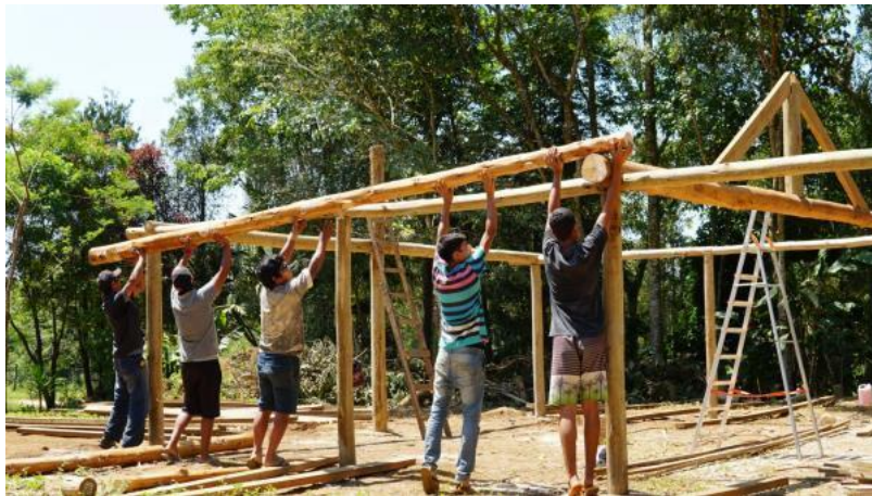
Figure 3. Construction of the new Prayer House, in the Tenondé Porã territory, 2020. Source: GTP Arquiteturas Tradicionais Collection
